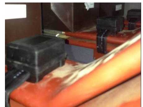
Sensor mounted on busbar
