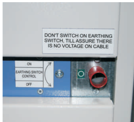
Mechanical indicator of earthing switch status
