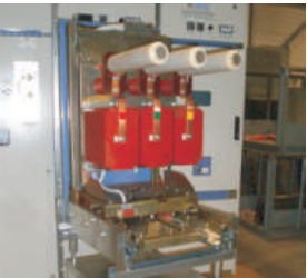
Voltage transformer on truck
