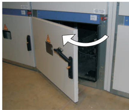
Opening cable compartment door
