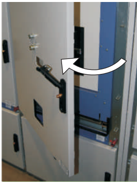
Opening draw-out element compartment door
