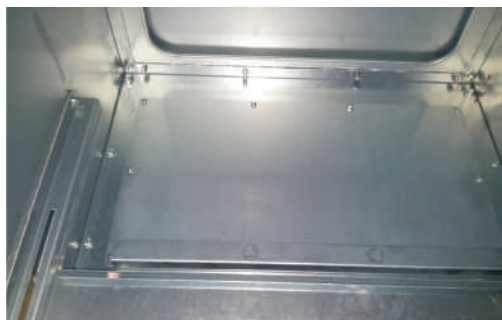
Removable access panel to busbar compartment
