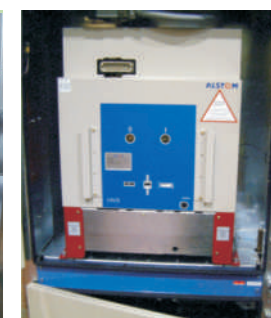
HVX Schneider Electric
